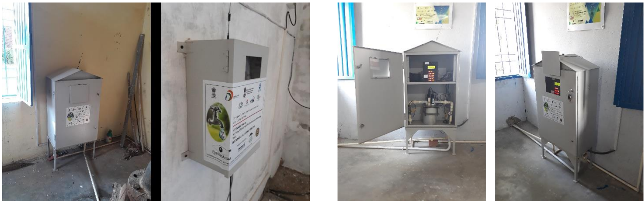
Real time water monitoring unit
