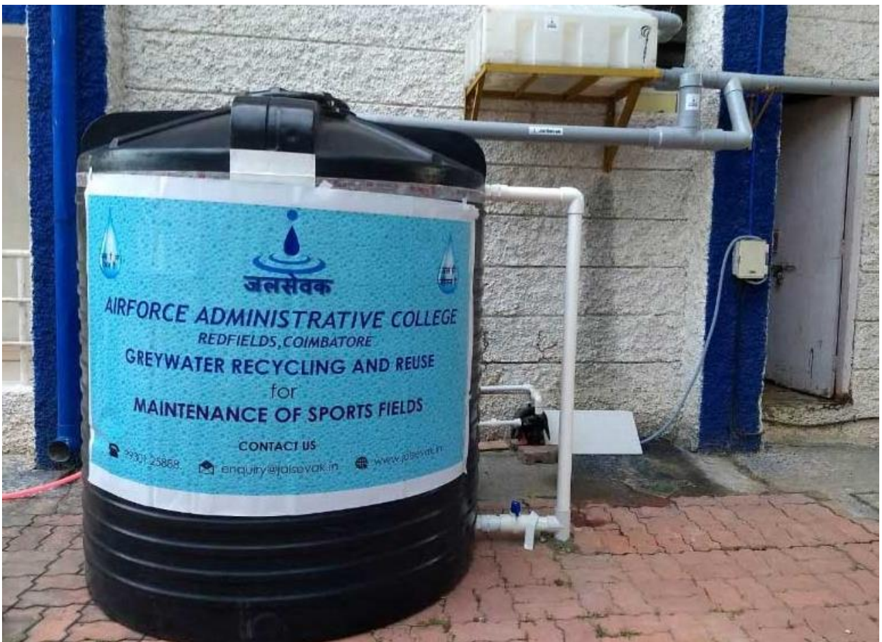
Pilot installation of devices to capture real time monitoring to reduce water loss
