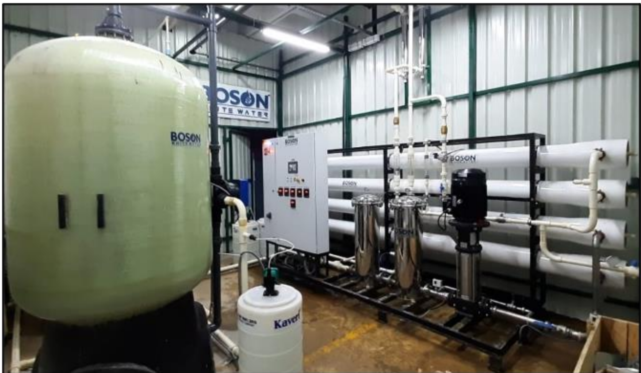
BOSON White Water System installation
