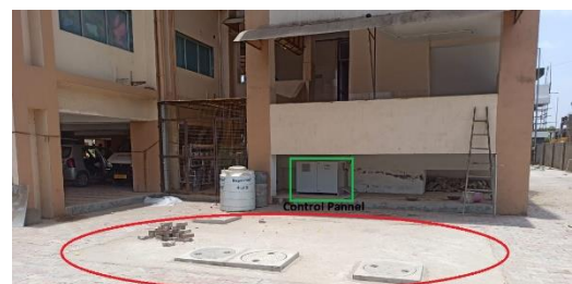
STP underground tanks
