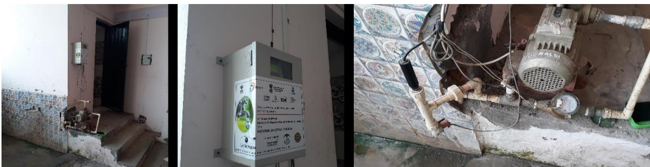
Installation of IoT based Water monitoring systems
