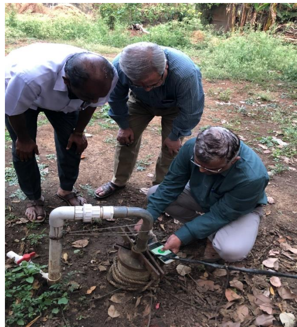
Installation of borewell monitoring app
