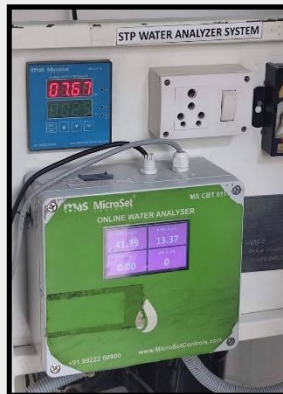
IT Park STP Hinjewadi, Pune FL-WQMS
