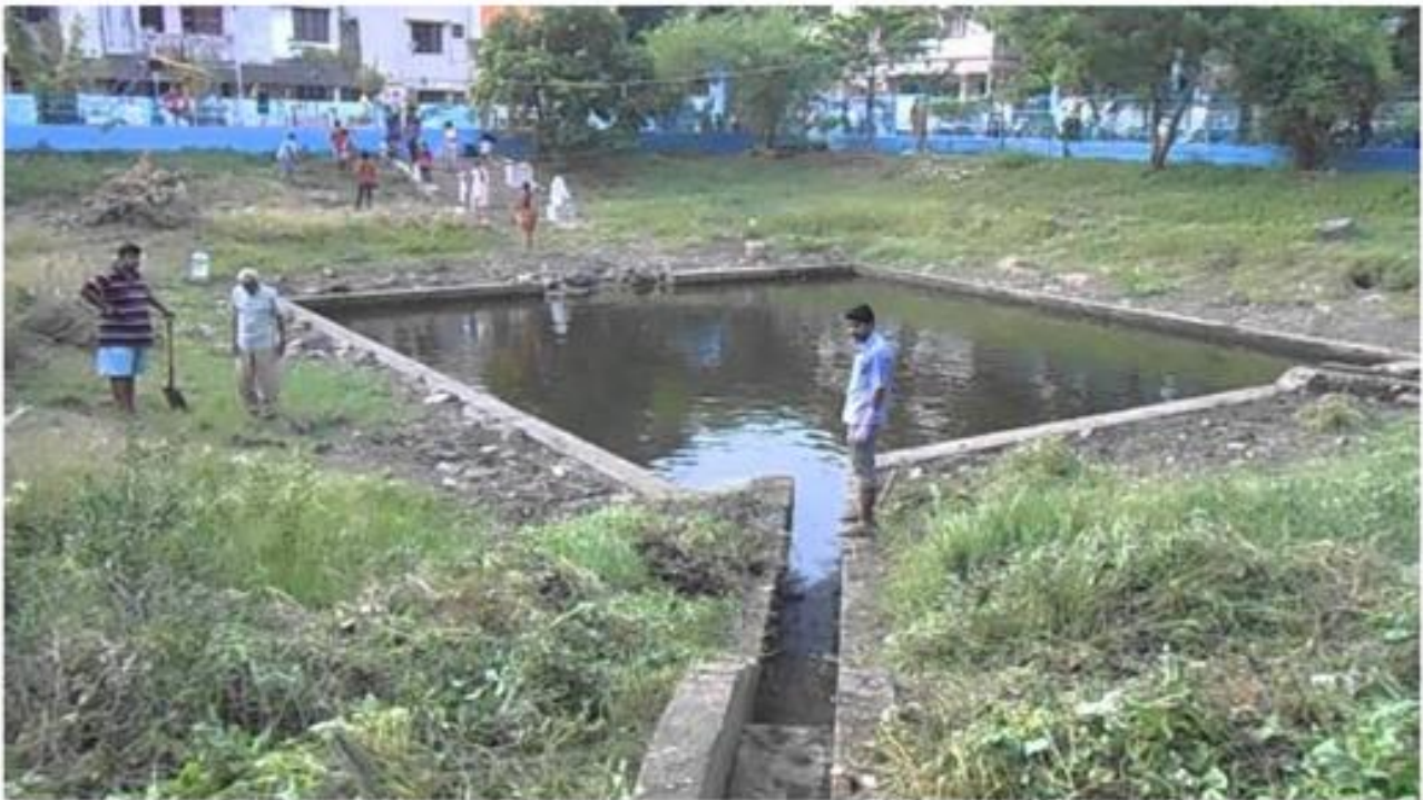
On – site rainwater recharging
