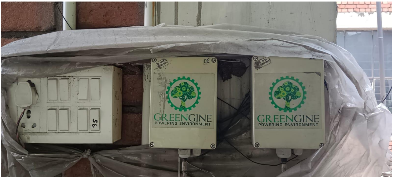
G- Water- I – digital water management system
