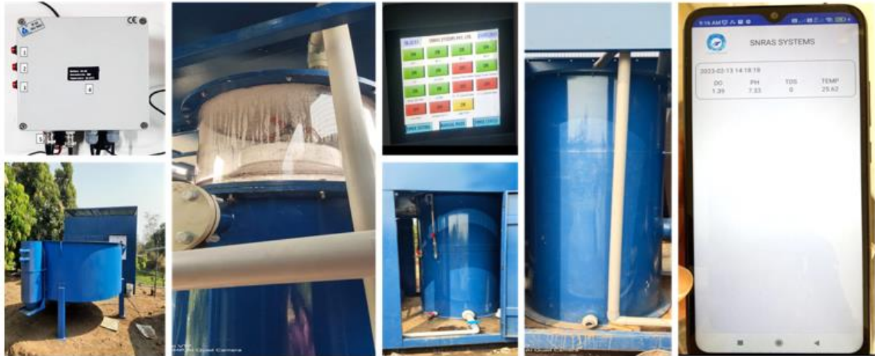
SNRAS waste water purification system infrastructure
