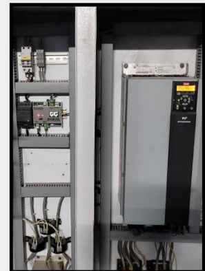
IT Park STP Pune DO Monitoring and Controlling
