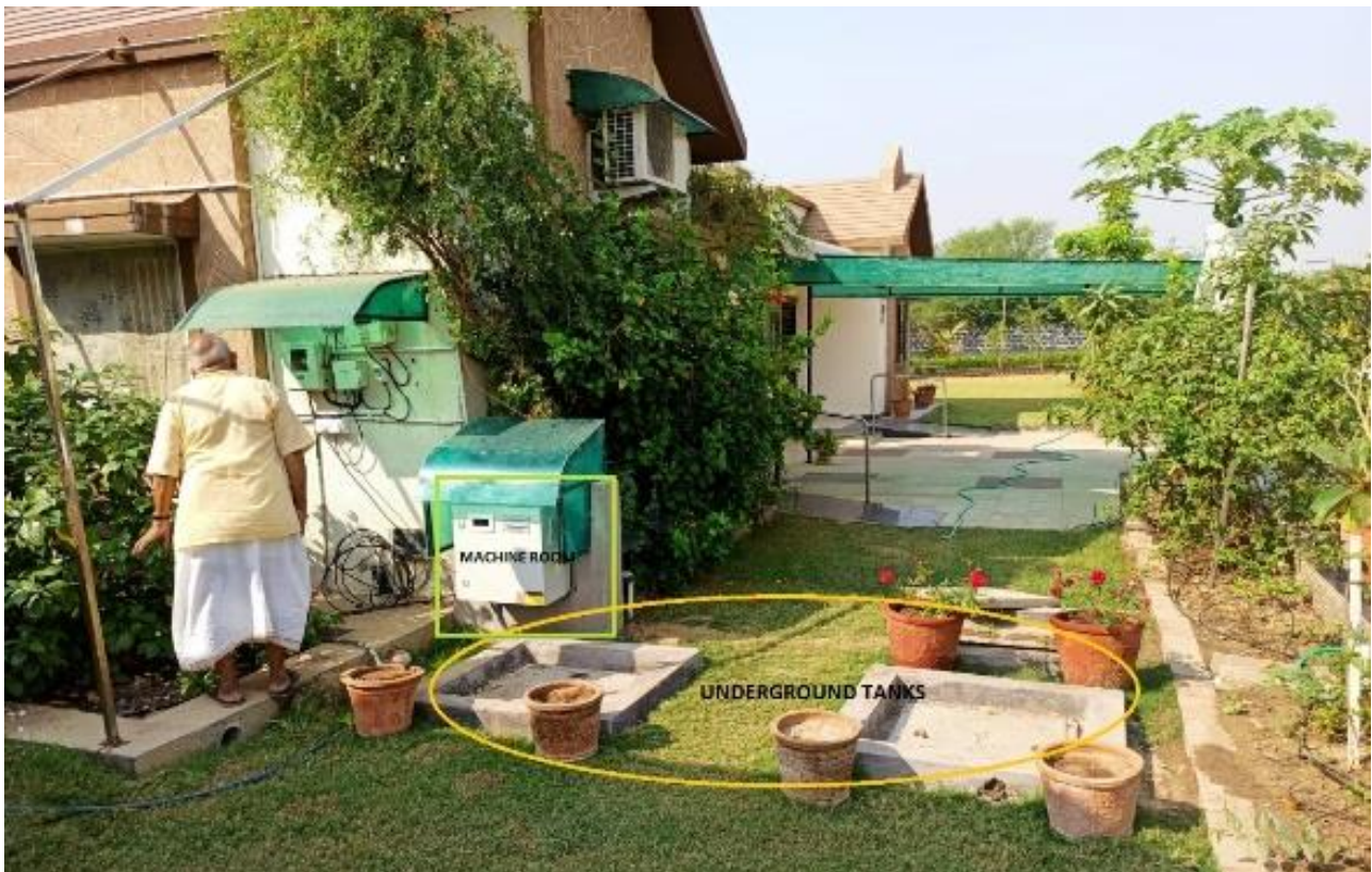
Sequence Batch Reactor-Sewage Treatment Plant at household
